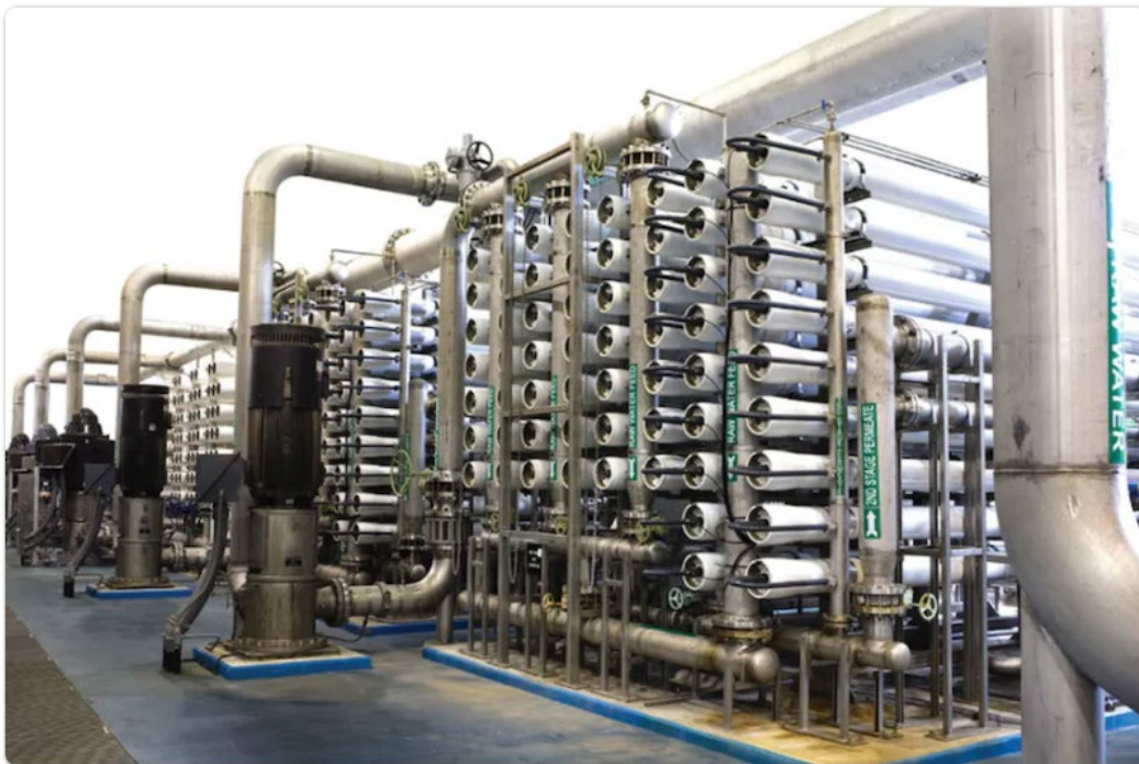
Figure 17-7: Reverse Osmosis Skid with Membranes
