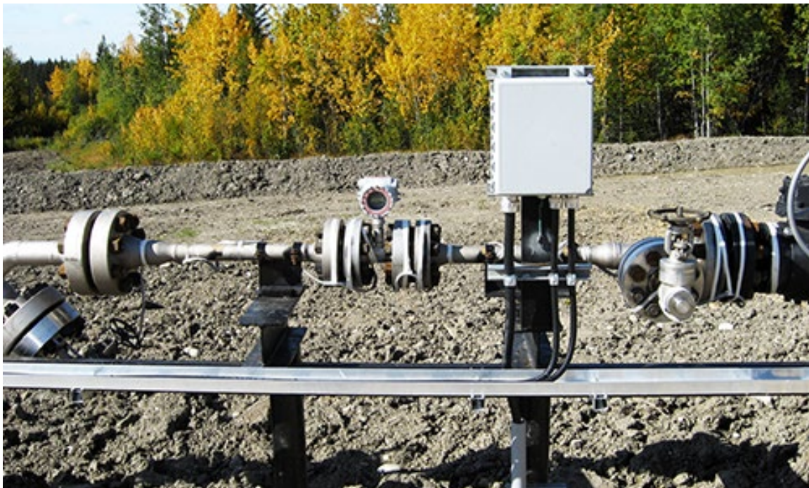
Figure 18-9: Pipeline Flow Measurement & Leak Detection System
