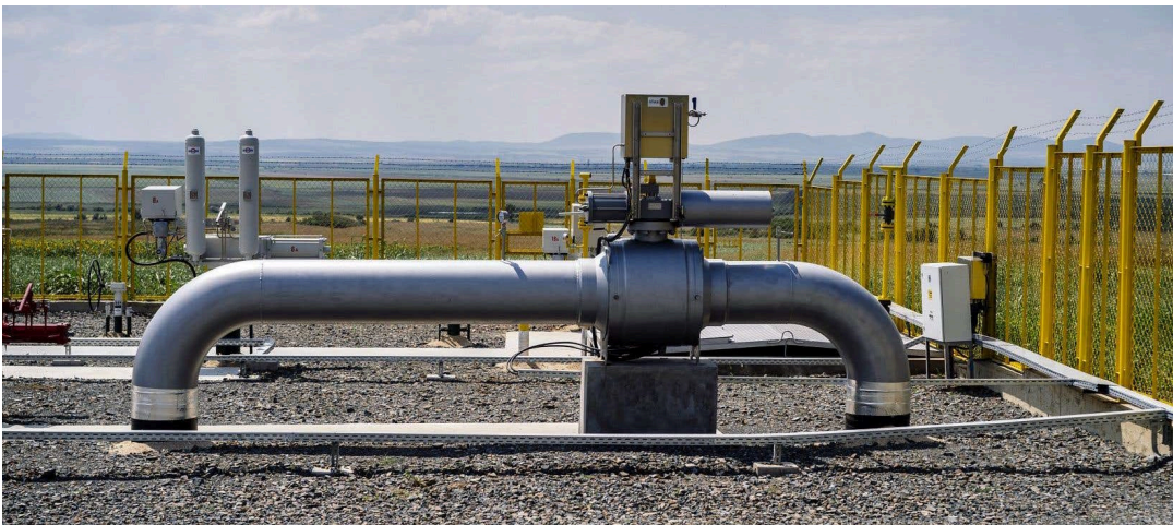
Figure 20-5: Field Example – Pipeline Riser
